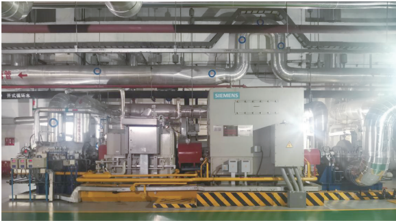
图 5 塔山电厂 1B 行星变频调速装置电动给水泵组 Fig.5 Electric feed pump set of 1B planetary frequenay conversion speed regulation device in Tashan power plant
